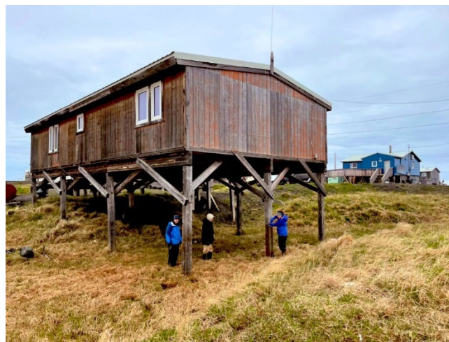
Figure 6: Point Lay home with pilings exposed due to ground subsidence. Ben Jones, 2022.
